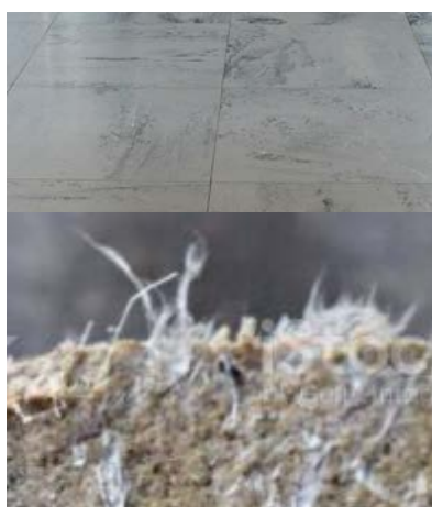
Figure 1: On top the picture of typical floor plates from today, below the view to the edge of an old floor plate with Asbestos fibres.
